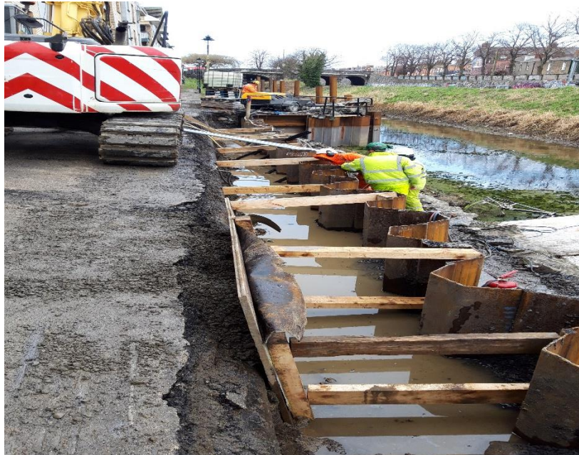
Hilliard's Engineering installing soil nails to support sheet piles opposite Portland Place Park
